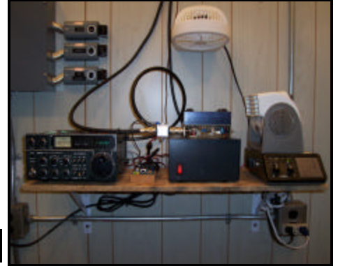
The Entire Beacon Setup With Cooling
